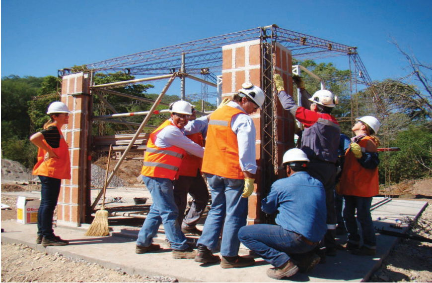
Construction of a housing unit using technologies developed by CEVE. Photo provided by Dr. Daniela Gargantini.
